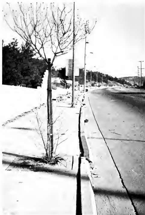
Photo 7. Damage to concrete block retaining walls, sidewalk, and gutter along Balboa Boulevard (west side).
